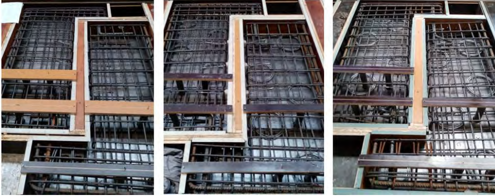
Figure 5-8 Wall panels before casting (from left to right: WL1T2, WL2T2 and WL3T3)
