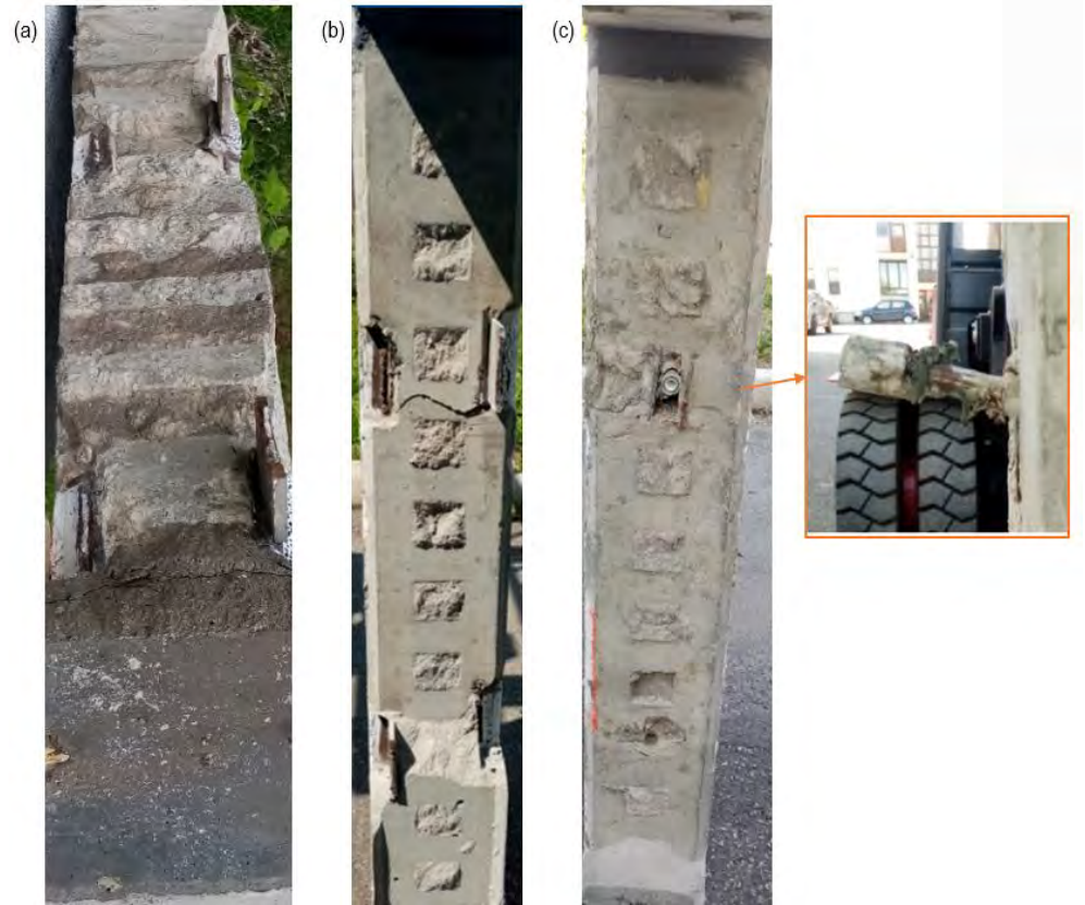
Figure 5-19 Steel assemblies specimens (SA1, SA2, SA3 series) after failure
