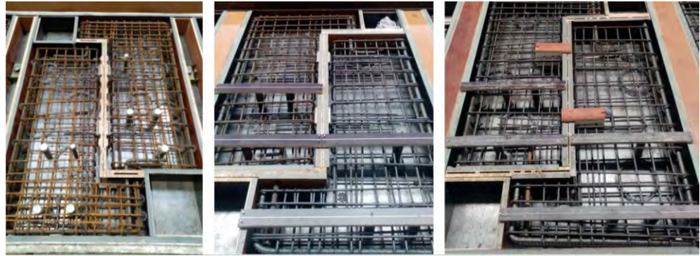
Figure 5-5 Wall panels before casting (from left to right: SA1T2, SA2T2 and SA3T3)
