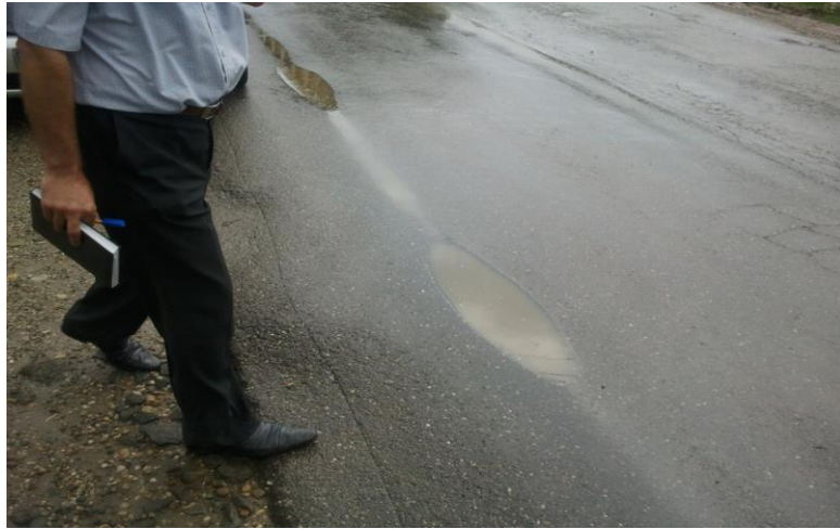
Figure 1. Deformation of asphalt layer due to poor compaction after pipeline intervention on DJ 108A
