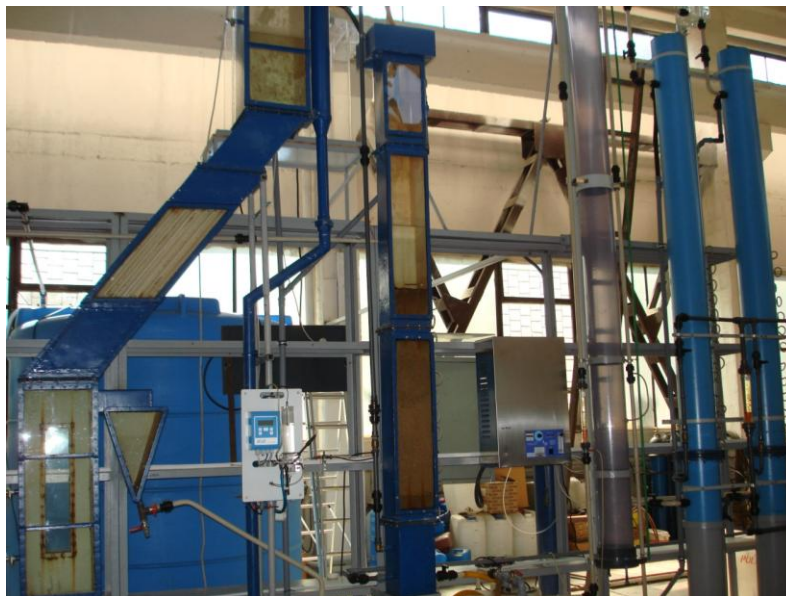
Figure 2. Water Treatment Pilot Plant, UTCB.
